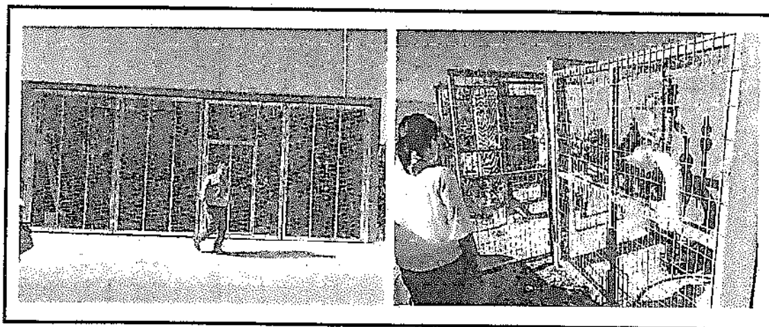
Pressure Reducing Valve (photos in JSC, Jenin)
