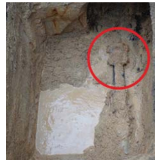
After digging the area, water leakage was identified.
