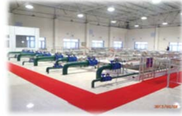
Large scale municipal water supply (40,000 m 3 /day)
