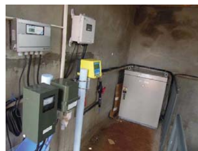
Photo1 Inside Monitoring Station
