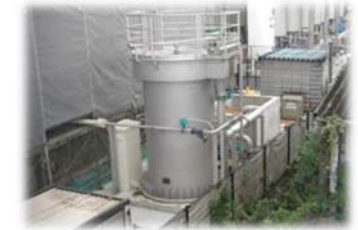
Stand-alone industrial water system ( food processing, linen, paper mill ) systems - various scales
