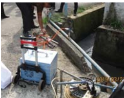
1. Injecting tracer gas
