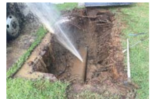
4. Leakage is found
