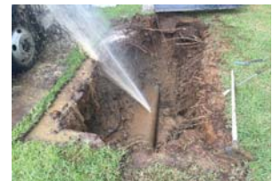
4. Leakage is found
