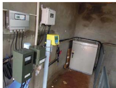
Photo1 Inside Monitoring Station
