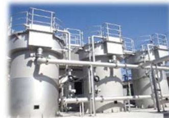
Compact design for municipal water supply system, medium scale (4,500 m 3 /day)
