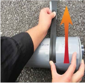
① After taking backpaper, apply tensor to Tomezo, cover the leak spot.
