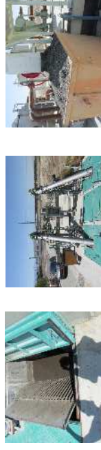
Screen and Grid chamber
