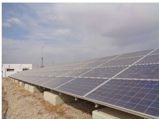
Photo -3 Solar Power Generation Facility
