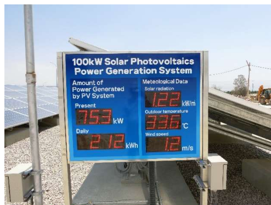
Photo -4 Generated Power Panel
