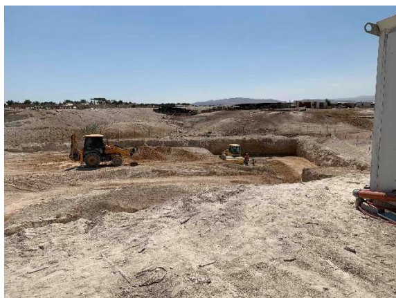
Photo 2.1.14 Pre-treatment Plant (Sept. 2021)
