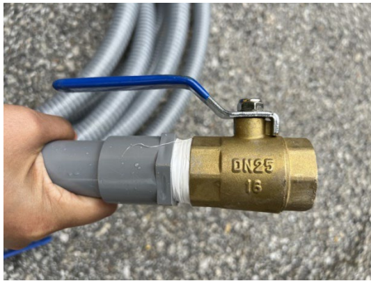
90. Valve connected to nozzle
