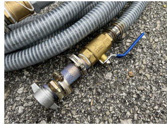
91. Valve connected to engine (if no valve it is okay)
