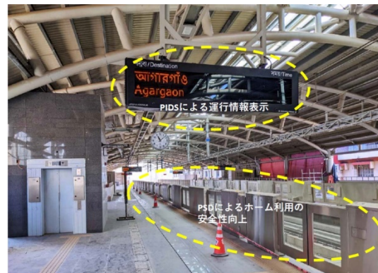
(ii) Example of ensuring accessibility for station and rail users: Passenger Information Display System (PIDS), and Platform Screen Door (PSD)
