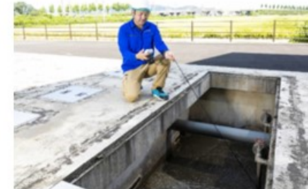
Settlement Drainage System
