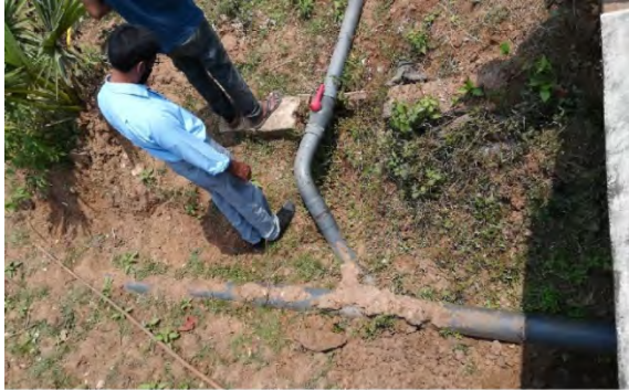
PVC Pipeline and Division Valve
