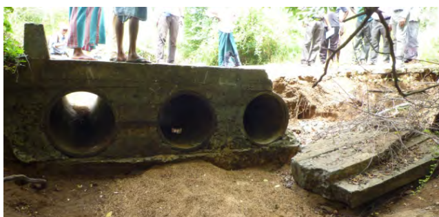
Source: PID Flood damage report
