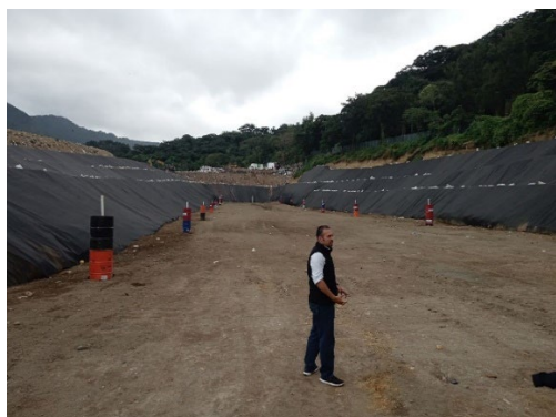
Sanitary landfill in operation. Guatemala's first project. The engineer who designed this repository was a JICA trainee.
