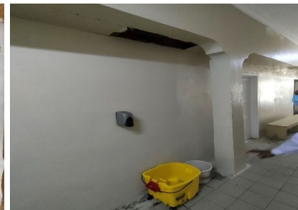
The facility has not been renovated since it opened, and is aging. The ceiling collapsed and there was a water leak.
