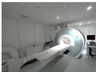
The MRI has never been used and has been left out of order. Not repairable
