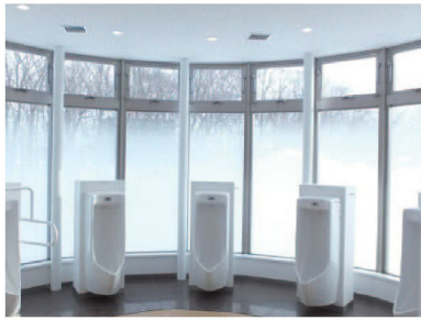
Toilets are in operation 24 hours a day. Clean, convenient toilets translate into increases in visitors to Michi-no-Ekis.
