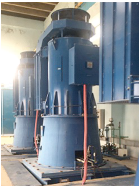
Drainage Pumps Installed under the Project
