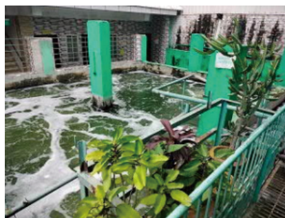
Wastewater treatment plant for a facility for cleaning garments for export, which was built with a loan from the Bangladesh Financial Sector Project for the Development of SMEs
