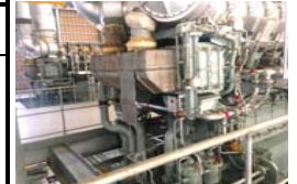
Please inform much more details of leakage point (start and wet/ accumulated)
