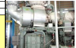
Smoke from lagging?
