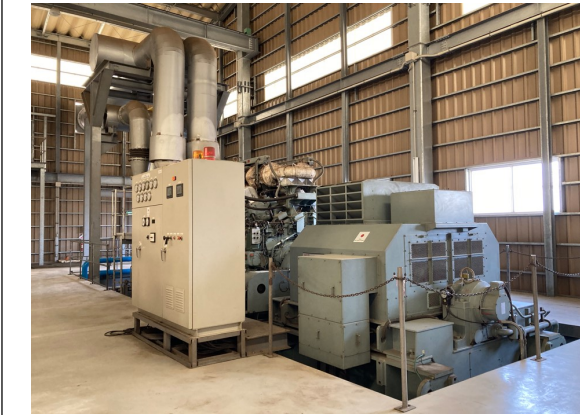
Diesel Generator Unit 1
