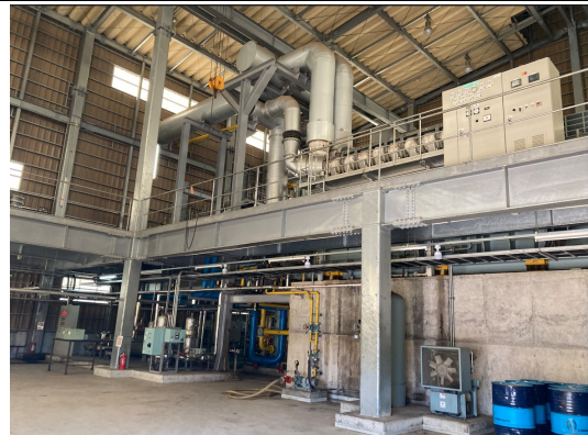
Power Plant (Interior)
