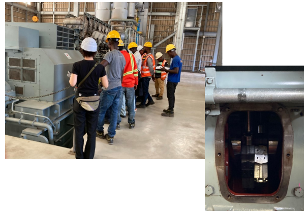
Diesel Generator Unit 2
