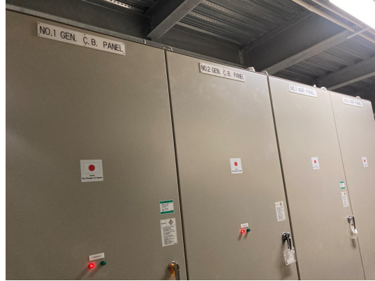
6.6kV Circuit Breaker
