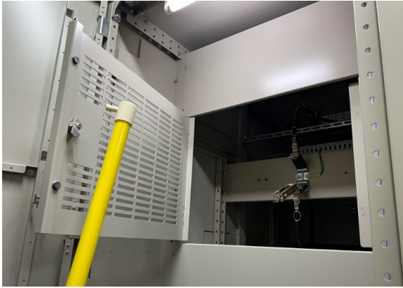
Disconnecting Switch for Neutral Earthing Resistor
