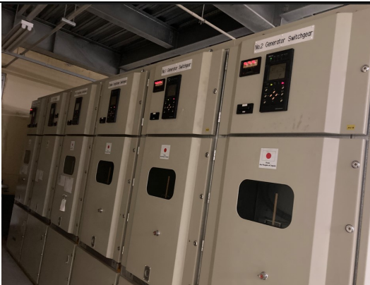
22kV Circuit Breaker
