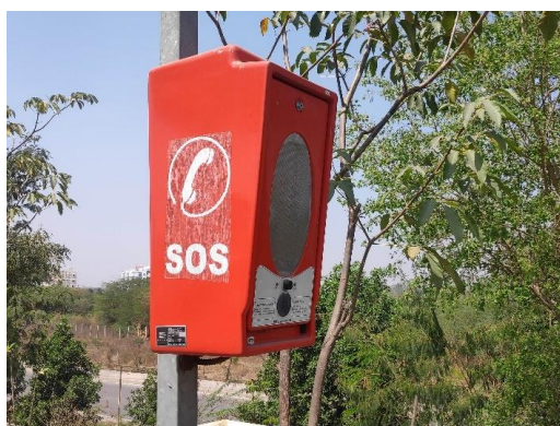
Emergency call box installed on the ORR
