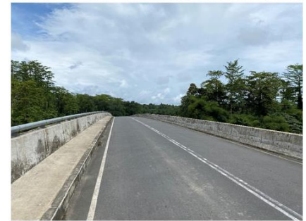
The bridges reconstructed under this project: Aum Bridge (above) and Kapiura Bridge (below) (Source: External Evaluator)
