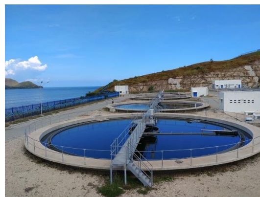
Joyce Bay Sewage Treatment Plant developed under the ODA Loan project (Source: Japan Economic Research Institute)
