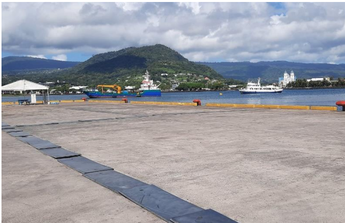
New wharf developed in this project (Source: Taken by the Local Associate)
