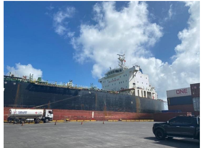
New wharf developed in this project and a cargo vessel in berthing (Source: External Evaluator)
