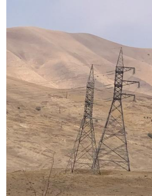
132 kV transmission line from Chwarta Substation
