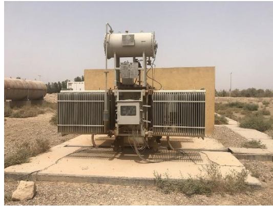
Transformer Installed under the Project (source: Ex-Post Evaluation Team)
