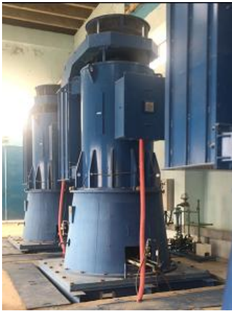
Drainage Pumps Installed under the Project (source: Ex-Post Evaluation Team)
