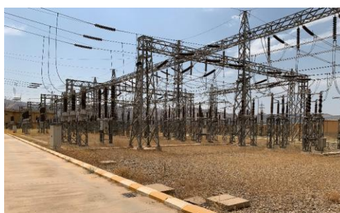
Chwarta Substation constructed under the project 2
