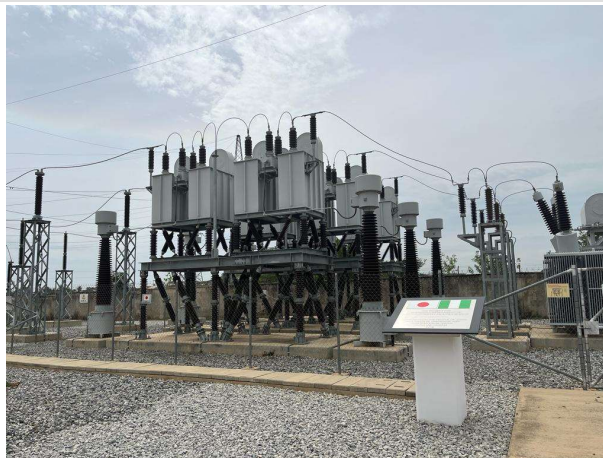
Power Capacitor Equipment installed in the Project (source: external evaluator)
