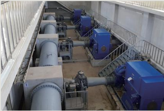
Transmission and distribution pumps installed by the project at the Nyaunghnapin First Phase Water Treatment Plant
