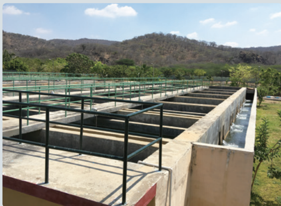
Hogenakkal Water Treatment Plant
