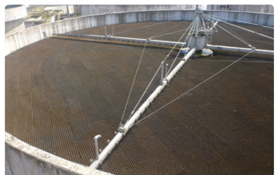
Wastewater treatment plant (trickling filter)
