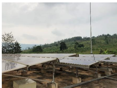
Solar panels for pump operation
