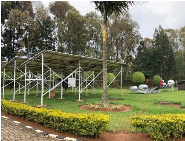
Solar water heaters/solar power generators (IPRC Tumba) (source: Taken by the Ex-post Evaluator)
