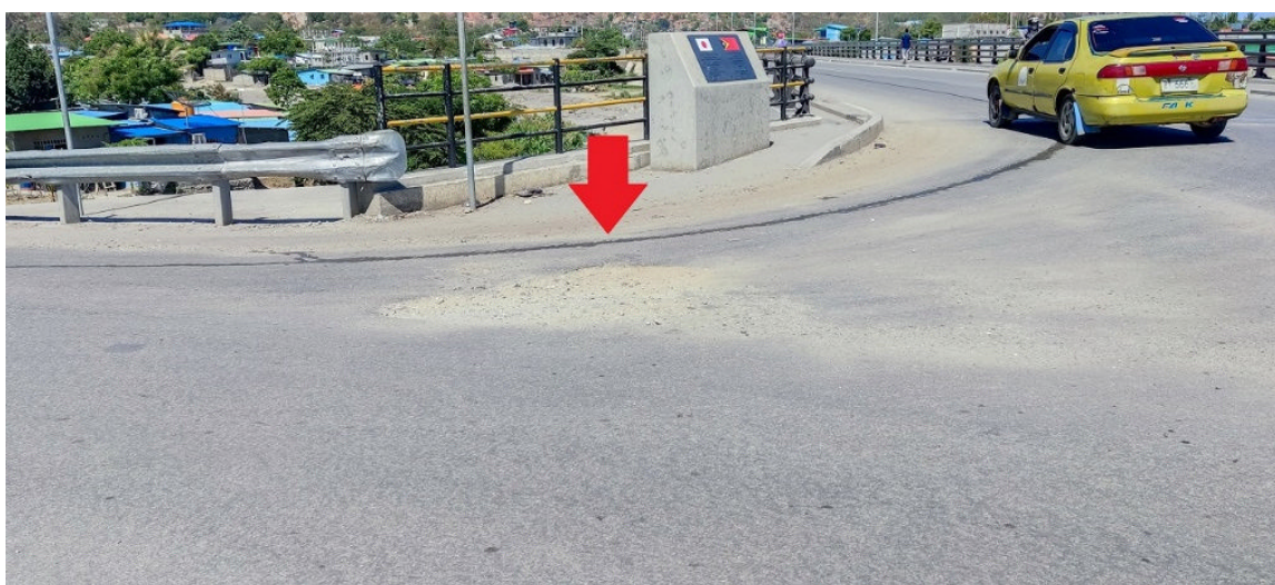
(Reference) Photo 8: Uneven Spots Near the Connection Between the Hinode Bridge and the Access Road (Sand lodged in the dent) (Photograph taken in October 2021)
