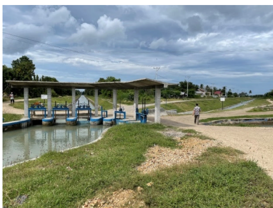
Branch Point of the Primary and the Secondary Canal (Mbay Kiri Subproject)
