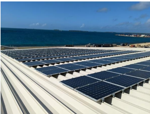
Solar panels on the roof of the passenger terminal building (Photo by External Evaluator)
