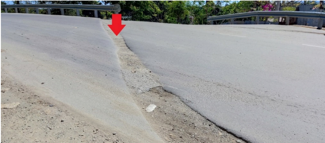
(Reference) Photo 9: Uneven Spots on the Access Road (Dent occurred) (Photograph taken in October 2021)
