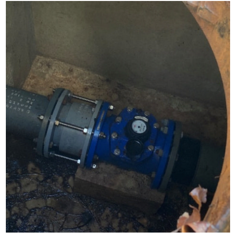
Flow Meter at Ngerkesoaol Service Tank Installed under This Project (source: taken by the evaluator)
