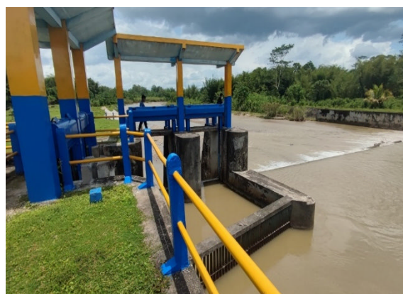
Developed Intake Weir (Way Apu Subproject)
