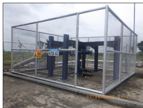
A well planned for CO 2 injection in the Gundih gas field
