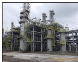
Natural gas production plant
