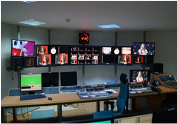
Photo 3: Master Control System for the TV Channels (Source: Tunisia Television Establishment)
