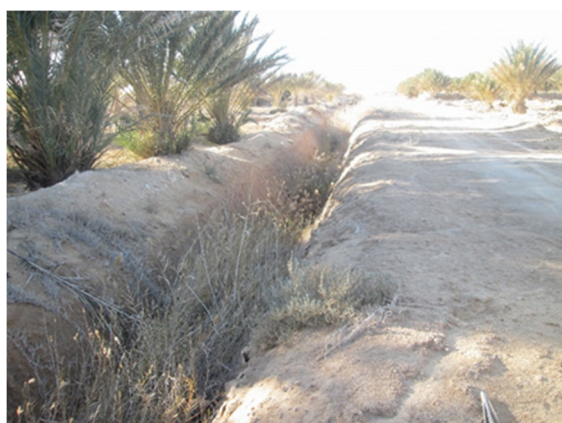
Photo 1: Developed Drainage Channel (Tabaga in Kebili Governorate)
