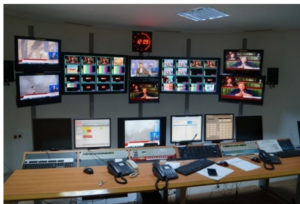
Procured Signal Distribution System (Source: Tunisia Television Establishment)
