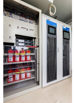
Inside of the VOR/DME (source: JICA)
