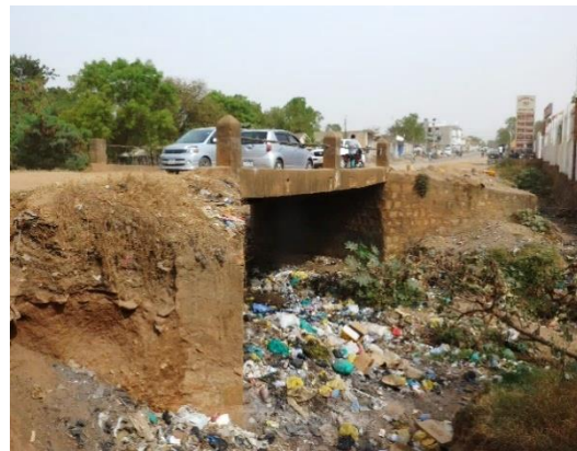
A river filled with waste dumped illegally
