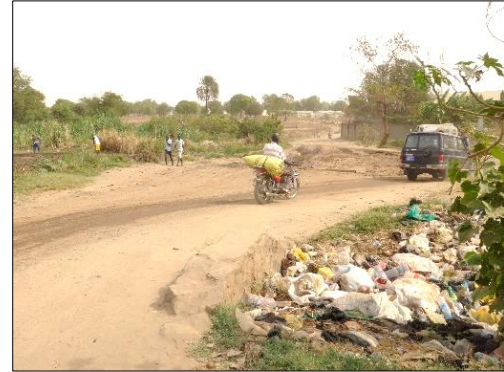
On the same road at the time of the ex-post evaluation, the culvert was filled with garbage, and the road was curved owing to sediment runoff. (February 2022) Source: Evaluator
