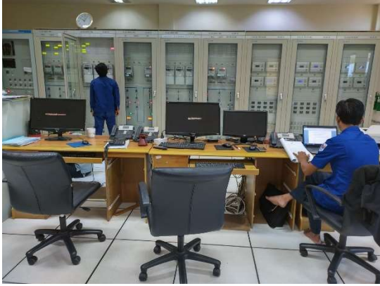
Control Room at Savaran Substation
