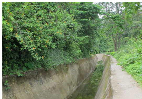
High Level Canal
