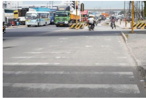
Road markings (markings faded)
