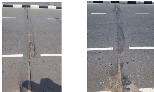
Before the repair work After the repair work Cracks on the pavement above the expansion joints (Kathaluwa bridge)
