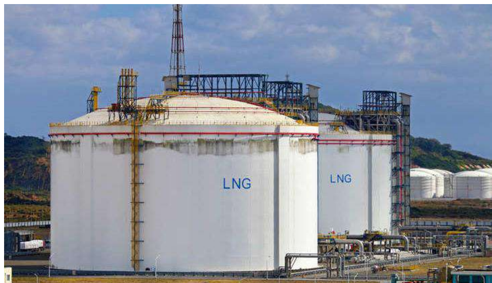
Exhibit 162: LNG handling at Mundra Port
