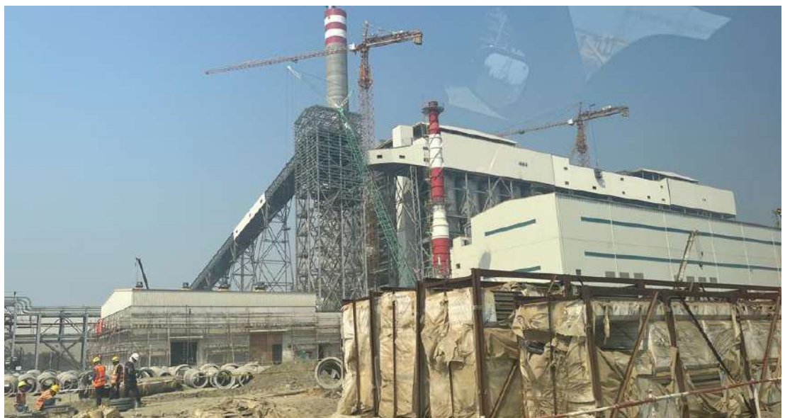
Exhibit 95: MIDI Site Pictures - Powerhouse
