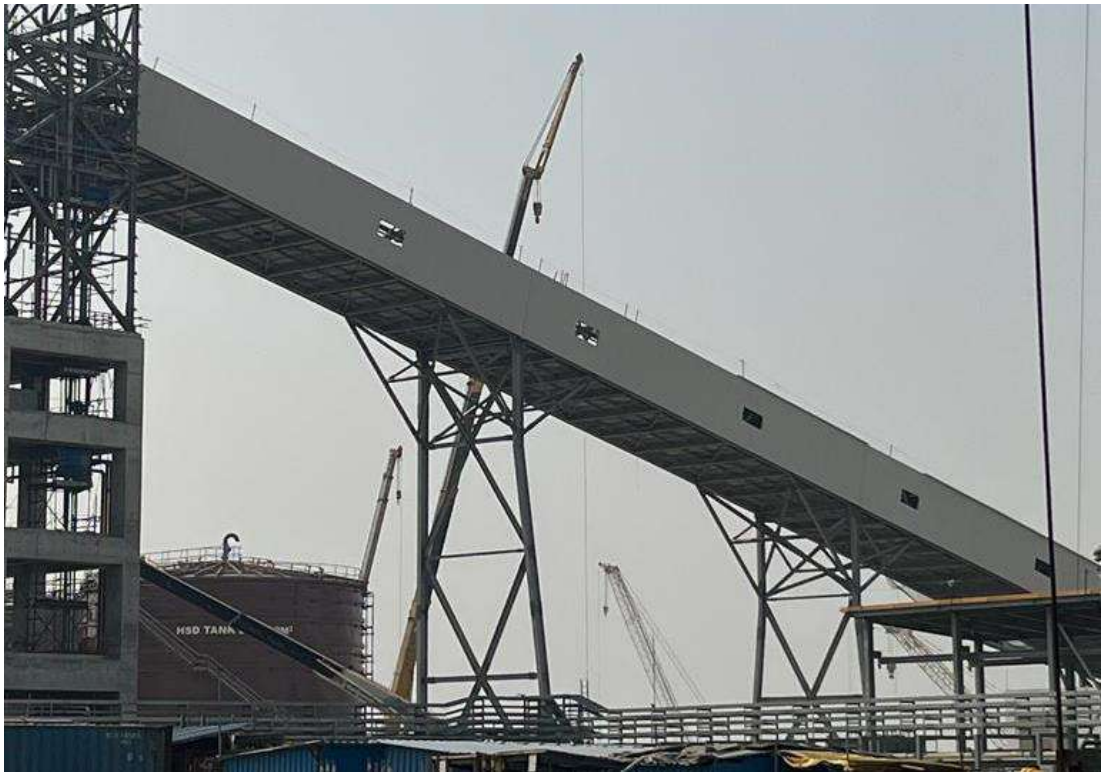
Exhibit 113: MIDI Site Pictures - HSD Tanks and conveyor belt (Power Plant)
