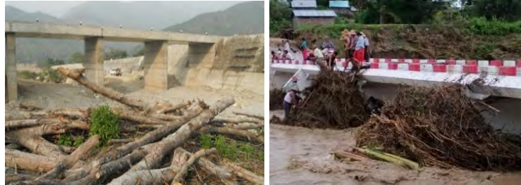
A case where log-shaped driftwood was confirmed on the upstream side of the box type causeway in the alluvial fan in hilly terrain.
