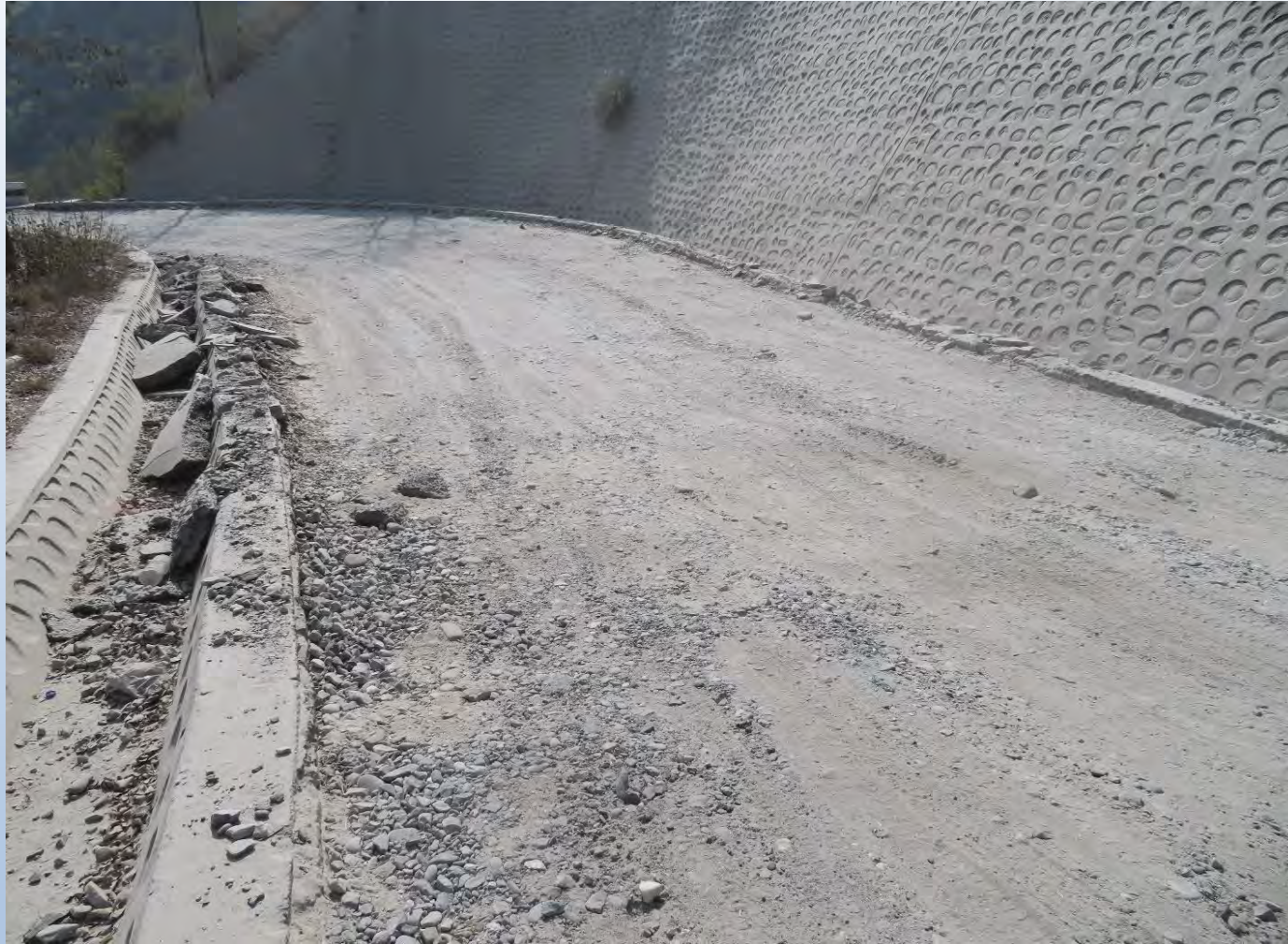
Removal of Asphalt Concrete for reconstruction at CH 93+900 to CH 93+500 (Sec. III) at Mulkot Bend
