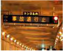
⑦ Warning Board in Tunnel
