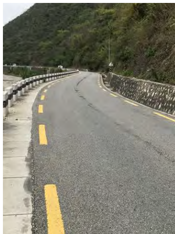
Peeled Surface at Road Center
