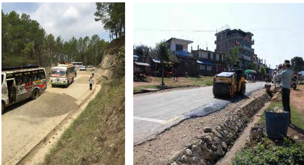
Figure 1.9 Site works with no traffic/safety control
