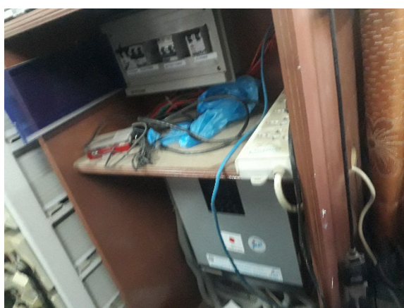
MCB switched turned off
