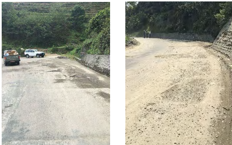
Figure 2.10 Entire Pavement Damage
