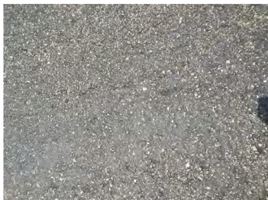
Minor Cracks on DBST
