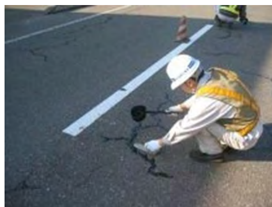
Image of Bitumen Penetration on Cracks
