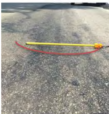
Rutting on Overlay
