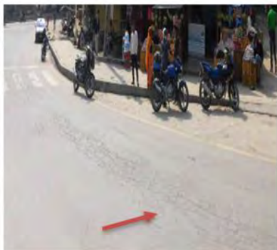
Alligator Crack Near Dhulikhel
