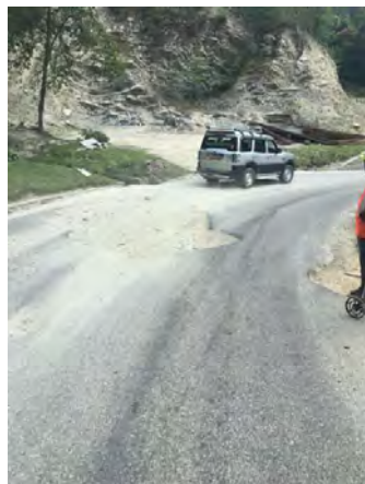
Pothole on Asphalt Overlay
