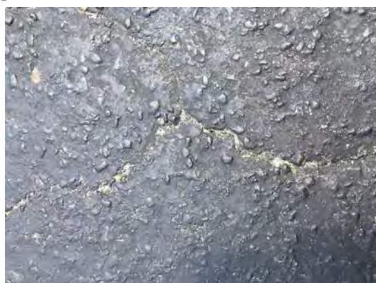
Cracks with 2 to 7 mm width
