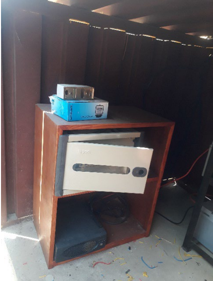
Battery and charger
