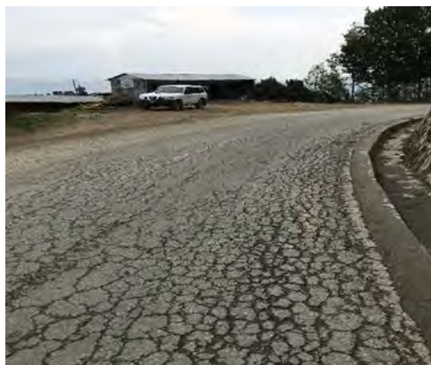
Advanced Alligator Cracks
