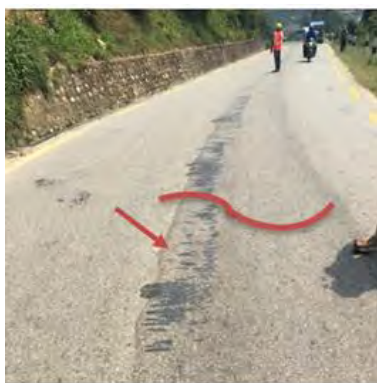
Rutting on Overlay
