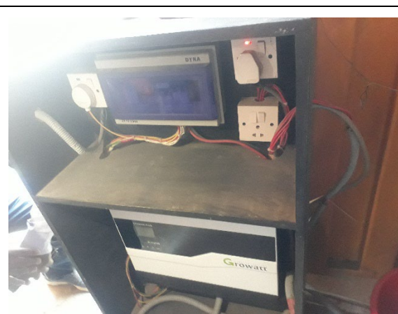
Inverter and switching inside control house
