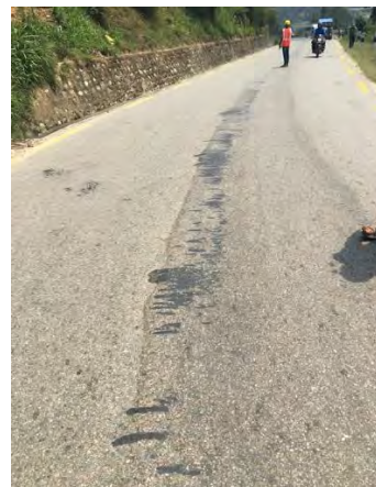
Rutting on Asphalt Overlay
