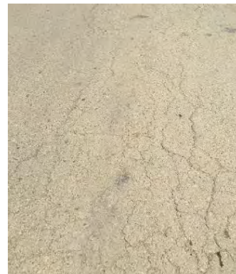
Alligator Crack Near Bhakundebsi
