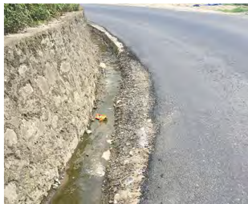
Unrepaired Side Drain After Overlay
