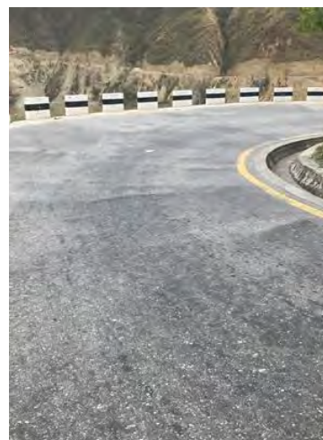
Rutting on Asphalt Concrete at Hairpin Curve at Mulkot
