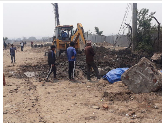
Road widening being carried out where there used to be control house
