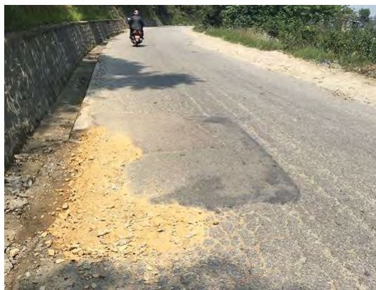
Damage of Side Drain
