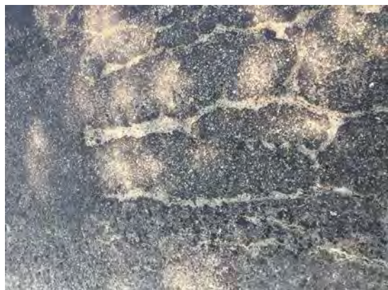
Cracks more than 7 mm wide
