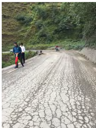
Alligator Crack on DBST
