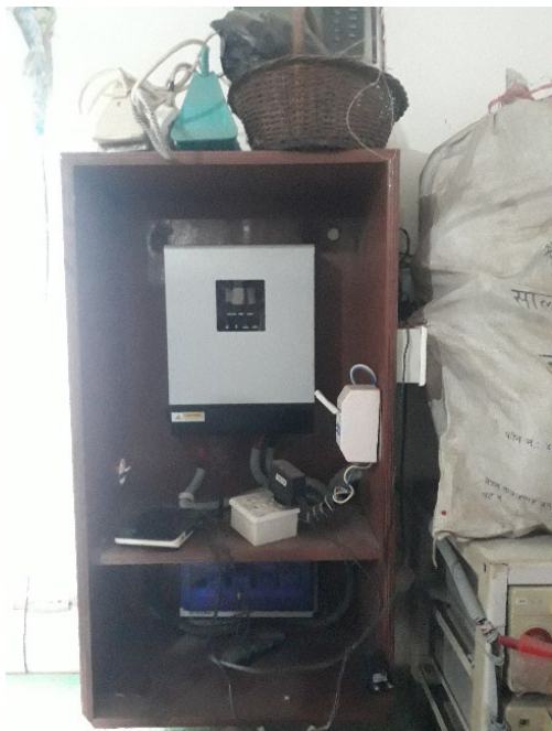
Inverter and electric connection at Bardibas rainfall station
