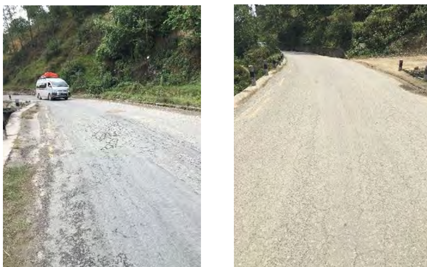
Figure 2.9 Alligator Cracks with Depression
