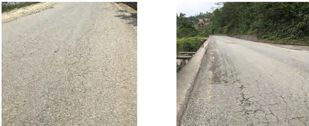
Figure 2.8 Alligator Cracks on Surface
