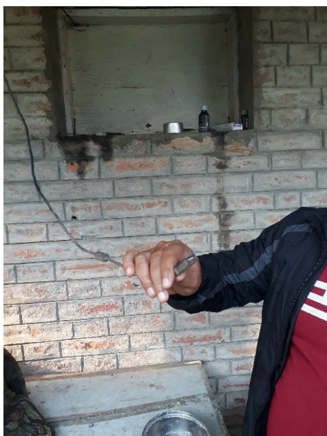
NCell Modem possibly damaged due to lightning
