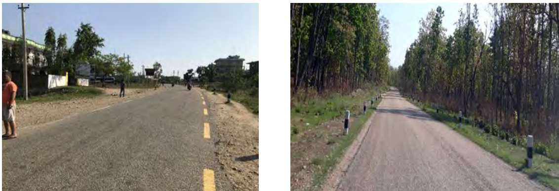
Figure 1.5 Pavement Conditions in Sec.I
