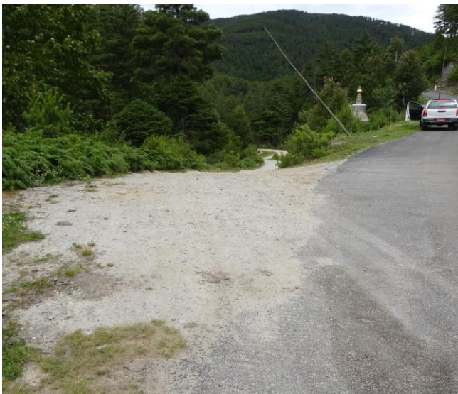
Farm Road constructed by using the procured equipment in Bumthang District connecting national highway, making easy access to the public facilities for the people of Chungphel Village.
