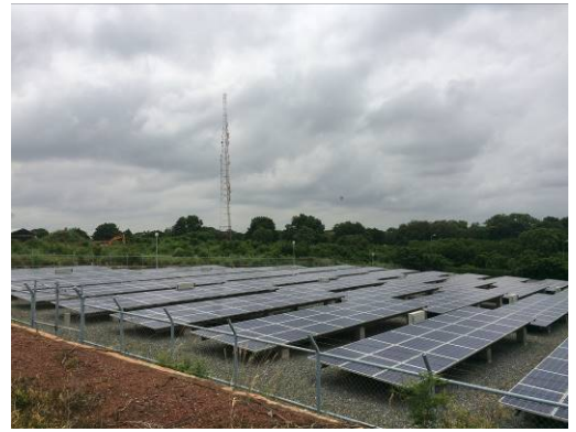
400 kWp Additional PV System
