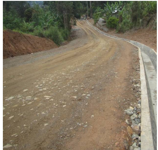
Fig 2: Road grading and maintenance work in Western Highlands Province using the procured equipment
