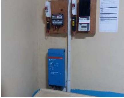
Well maintained PV system in South Horr Dispensary, Samburu County
