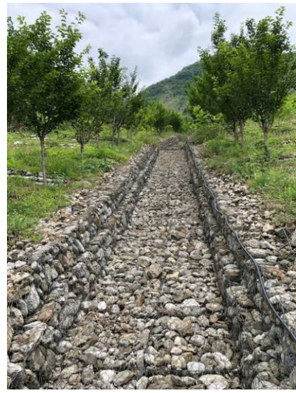
Independent construction site using the technology of the project in Beichuan County (constructed during the project period)
