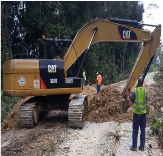
Fig 1: Disaster restoration work in Southern Highlands Province using equipment lent by Western Highlands Provincial Works
