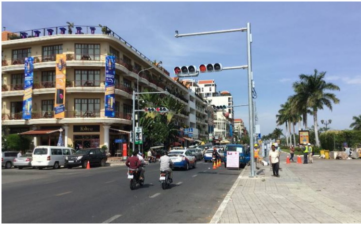
Installation of new traffic light system at one of intersections in Phnom Penh
