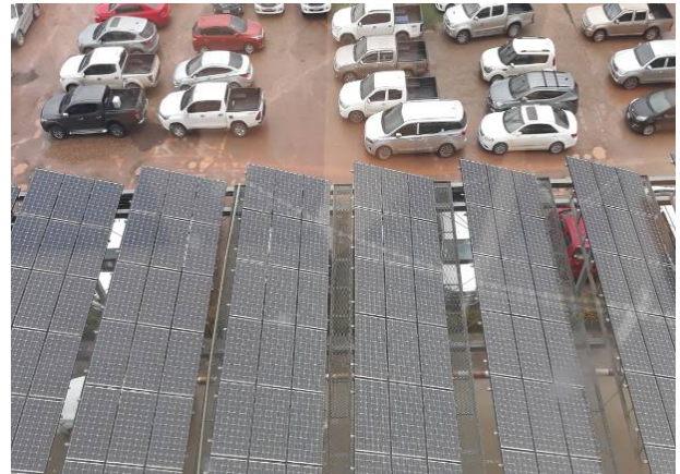
(Top view of PV system)
