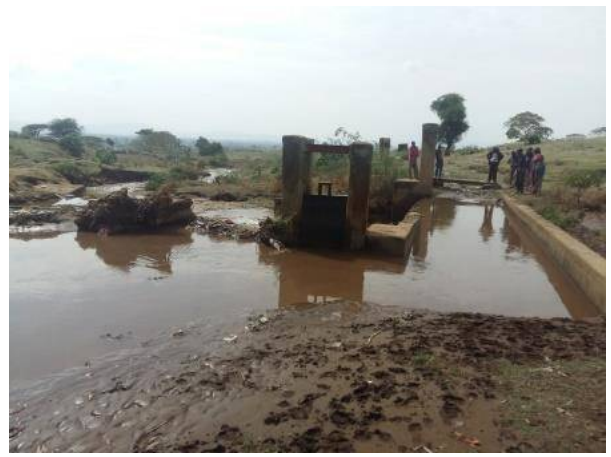
Burra irrigation site (Non-Functional)
