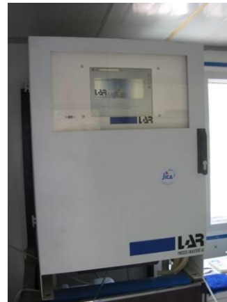
The toxic sensor installed in the upper stream area of Heihejinpen Dam Lake. No failure occurred since installment.
