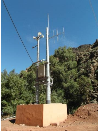
Tazitounte alarm station in Ourika valley
