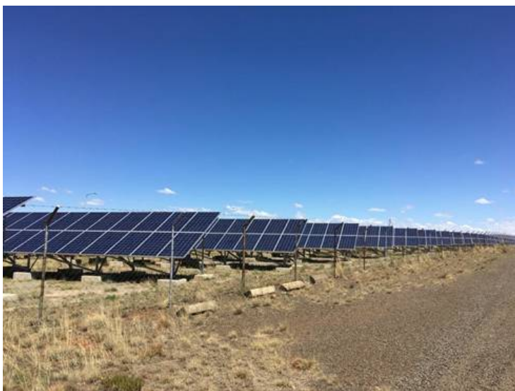
PV panels installed at MIA
