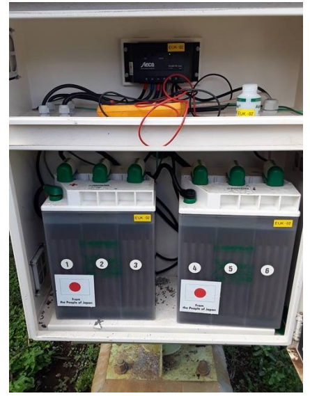
SHS box clean and well kept
