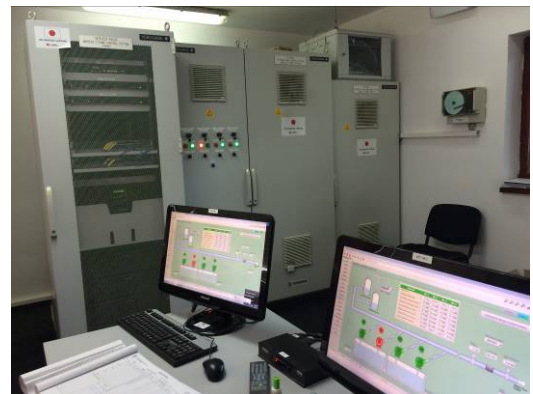
Monitoring room at Mareza 2 pump station
