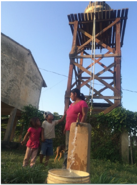
(Water facility with the solar Panel System in Puerto GERALDA Community, Beni)
