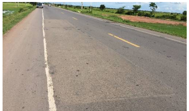
Maintenance Works for the National Road 6 in Siem Reap (between Krong Serey Sophoan to Krong Siem Reap)
