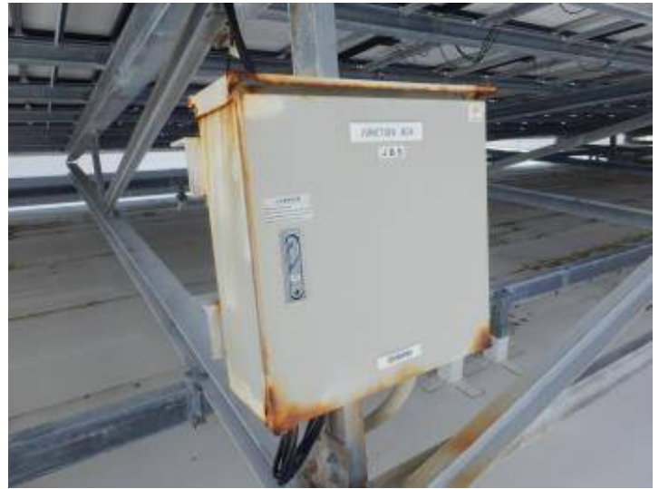
A junction box
