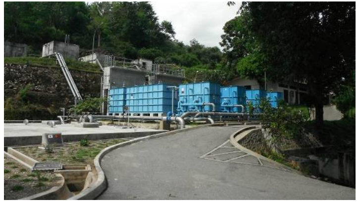
Bemos Water Treatment Plant Facilities
