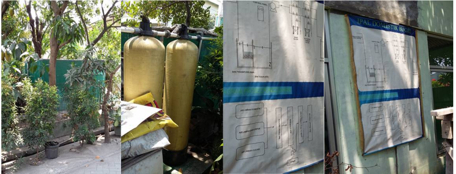
Communal wastewater treatment plant
