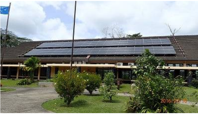
The PV system on the roof of the president office in the Federal Government Complex
