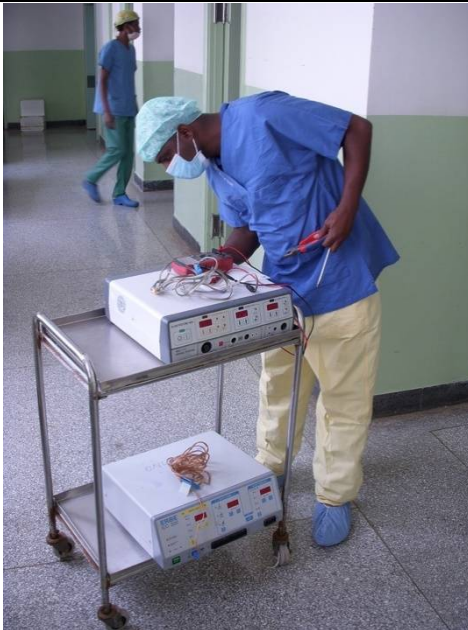
Technician inspecting ME of the surgical treatment room (Orotta Hospital)
