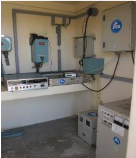
Equipment provided under the project (water level telemetry subsystem)
