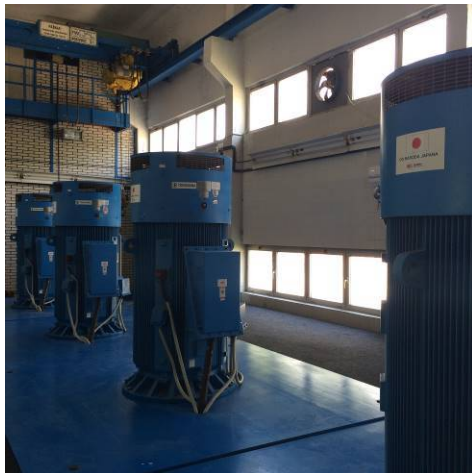
Four pumps at Mareza 2 pump station
