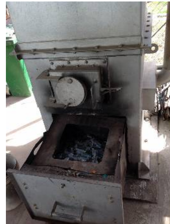
(Incinerator at Siem Reap RH)
