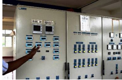
(Upgraded Equipment of Logwood Water Treatment Plant)
