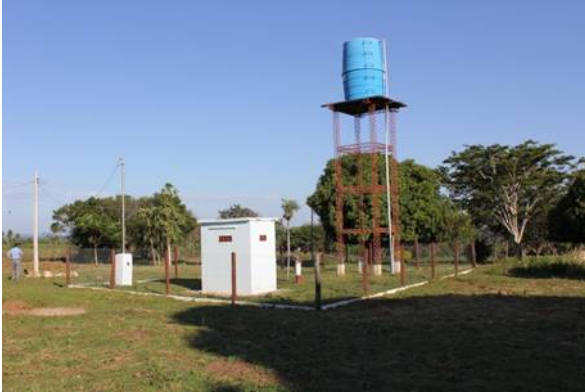
Nuahi Village, Achay Municipality, Paraguari Province (One of the 25 prioritized villages) Completed deep well drilling and water supply facilities
