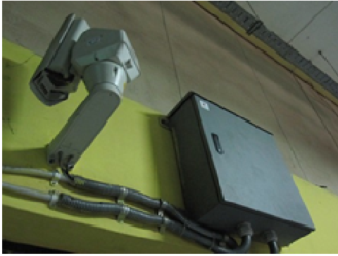
( Broken CCTV in Belawan port )
