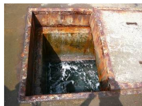
The malfunctioning hatch due to rusts on the metal part
