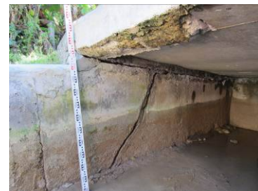
A crack on a side wall portion of the aqueduct under the bridge
