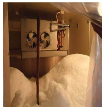
Ice plant with the ammoniac refrigeration system
