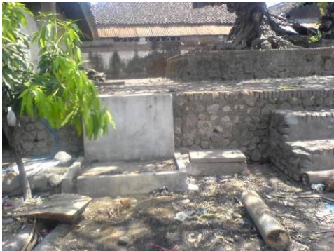
Unrepaired Public Tap
