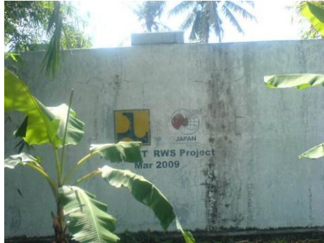
Water Reserve Tank
