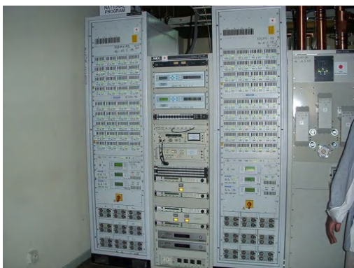
Transmission Equipment for Ngaoundéré Station
