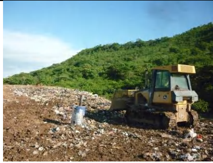
Provided equipment in operation
