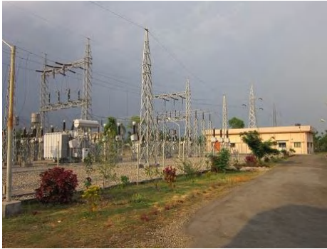
External View of New Kawasoti Substation
