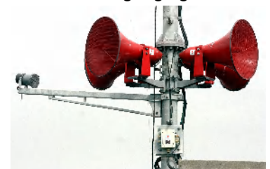
(PMD) Warning system (TMA)
