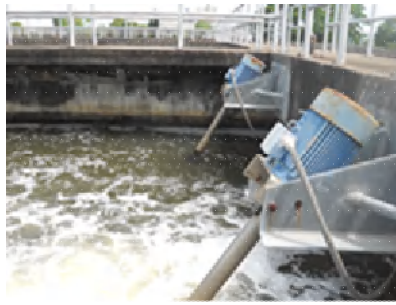
Aeration Tank at STP
