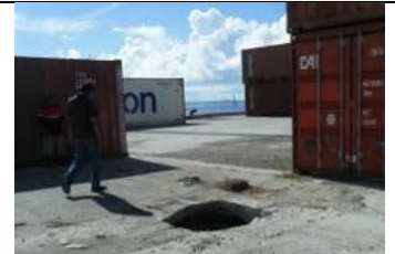
Cavings identified at the container yard
