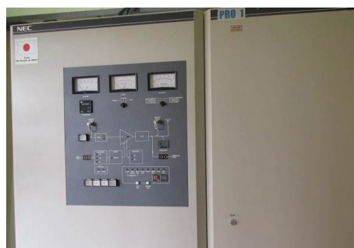
Transmitter Equipment for medium wave radio
