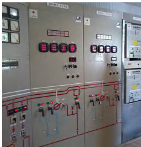
(Control panels for main transforms in the control building)
