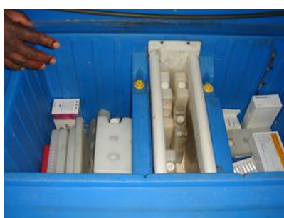
Well-organized and maintained solar refrigerator (at a health center in Chongwe)
