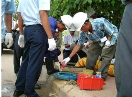
OJT on the maintenance of distribution facilities
