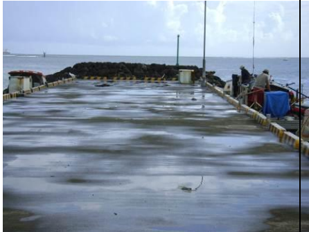
Revetment constructed during the project implementation to protect the port from high tide water
