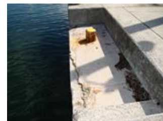
Partially delaminated concrete
