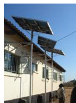
Solar panel for solar refrigerator
