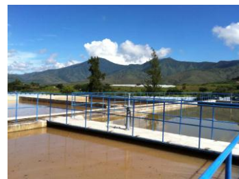
Slow filtration system in Salamá
