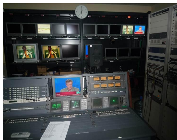
Main Control System replaced by the Project
