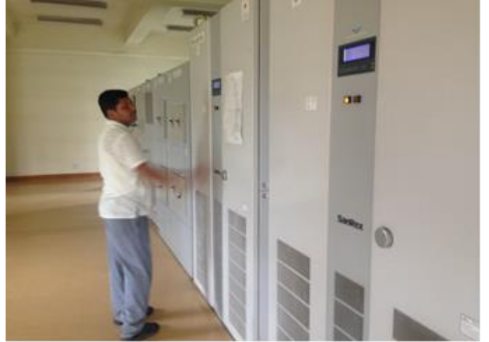
Solar Power Conditioner working properly
