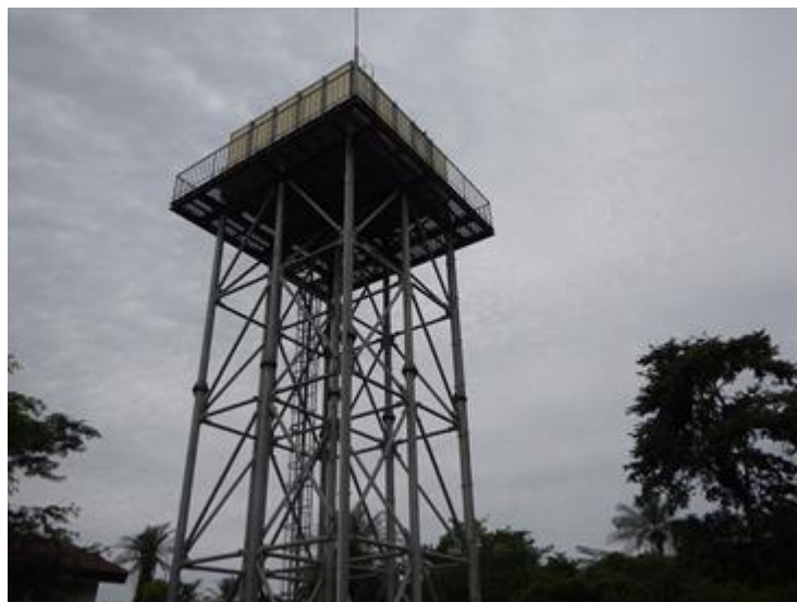
Water Reservoir on Tower in Cacine
