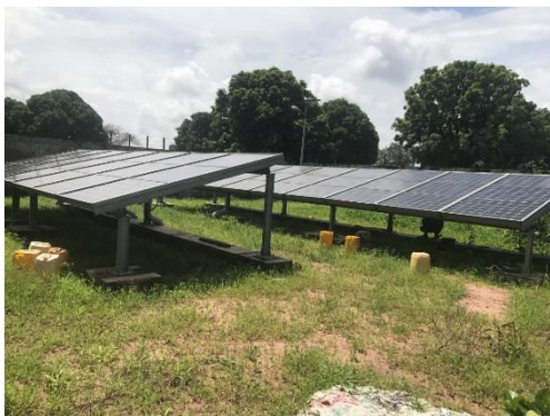
Solar panel of the water facility
