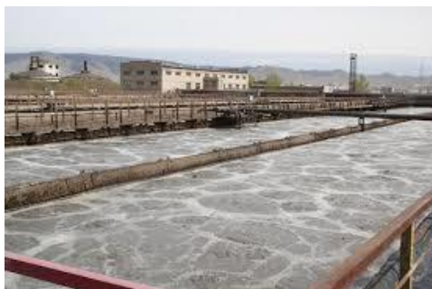
Current situation of the Central Wastewater Treatment Plant (at the time of ex-post evaluation)
