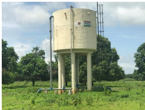
Water tank of the water facility
