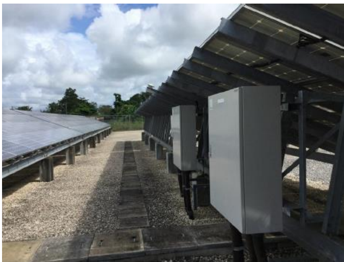
Solar radiation sensor and panel array
