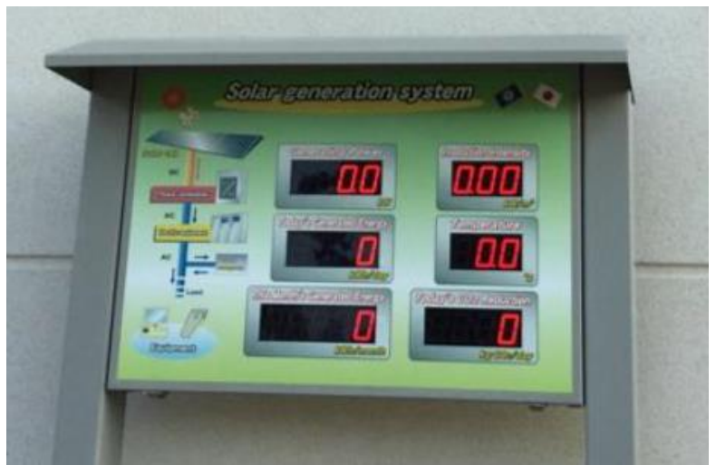
Monitor showing zero due to the broken data system
