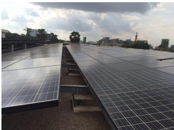
Solar panels on the roof of Phum Prek Water Treatment Plant
