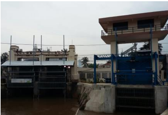
Additional gate at Manggarai Water Gate Point to increase the river flow capacity from 330 m 3 / sec to 570 m 3 /s.
