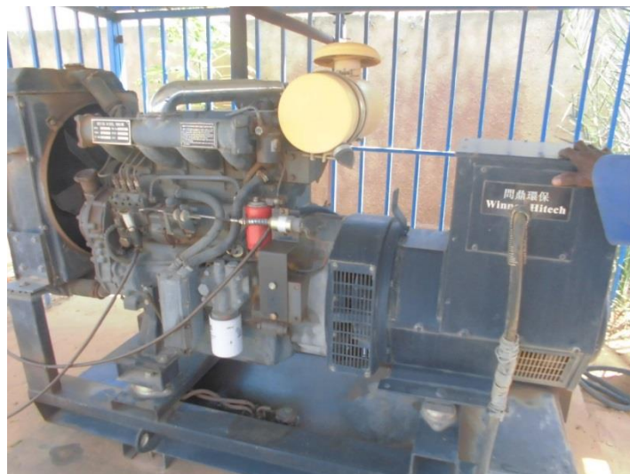
Generator used by SEEN on the site of Libore (Tillabery region)
