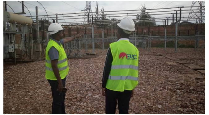
EUCL Engineers conduct regular patrol and inspections of the entire transmission system
