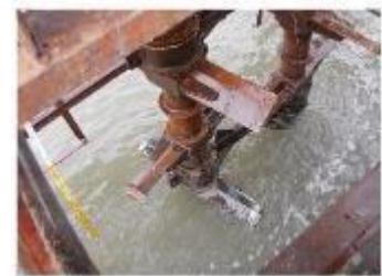
Source: Penta-Ocean Construction Ground improvement applying CDM (Thi Vai General Cargo Terminal)
