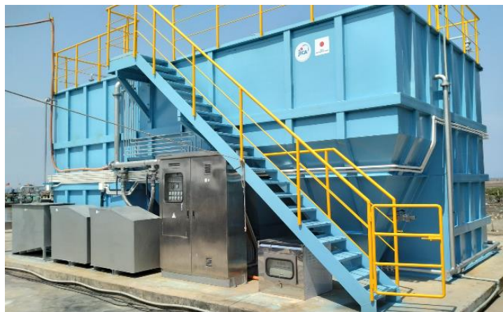
Fig. Equipment appearance (Installed at Ngoc Hai Seafood Market)
