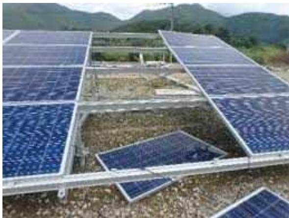
An example of PV panels damaged by a typhoon
