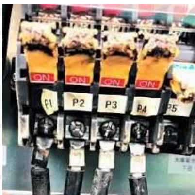
Burned PCS (Terminal box)
