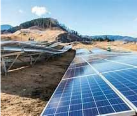
An example of Landslide PV array where on loose ground
