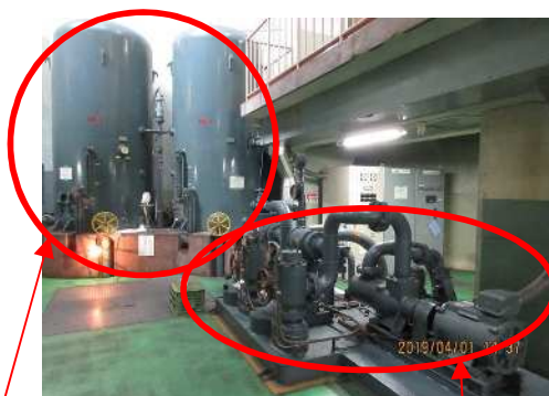
Pressure oil tank
