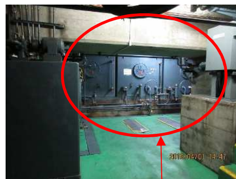
Oil collection tank
