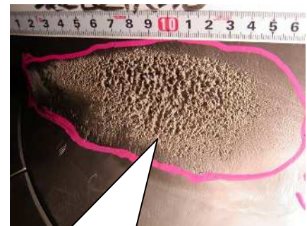
Roughness on the surface is a mark of cavitation erosion
