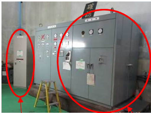
Governor Control Panel (Regulator)
