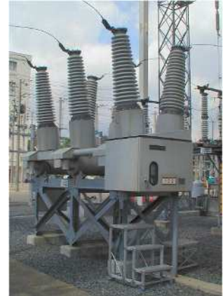
Circuit breaker type by rated voltage (Japanese case)
