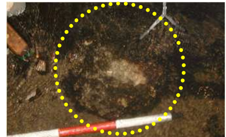
Local scouring by sediment
