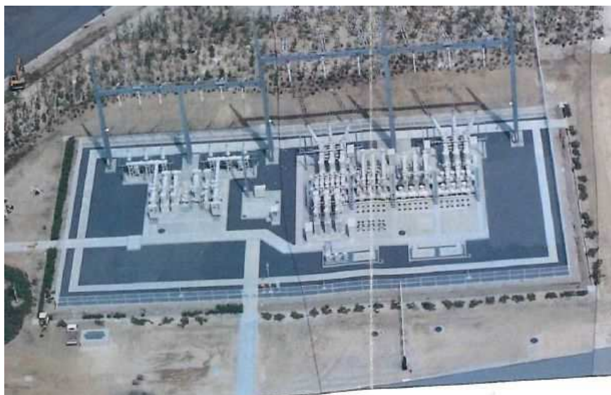
Photo. Switchyard in Yanai TPP
