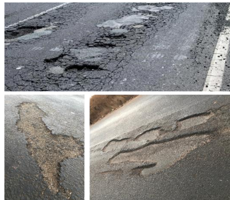
Photo 1: Damaged roads (National Route 1, Dakar Region)
