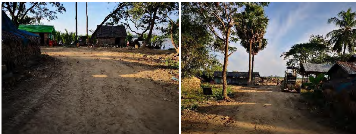
Existing access road from riverside to plant yard was widened and made good by MOC
