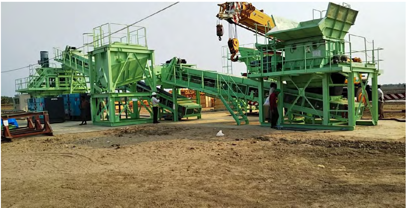
Placement of Screw Feeder (SF) for input of additive in position done
