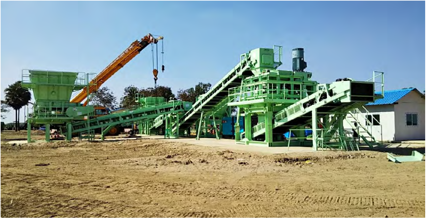
Placement of Apron Feeder (APF) & Cohesive Soil Feeder (WSF) in position done
