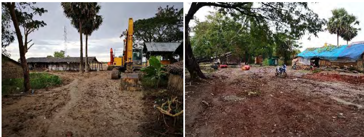
Existing access road from riverside to plant yard was widened and made good by MOC.
