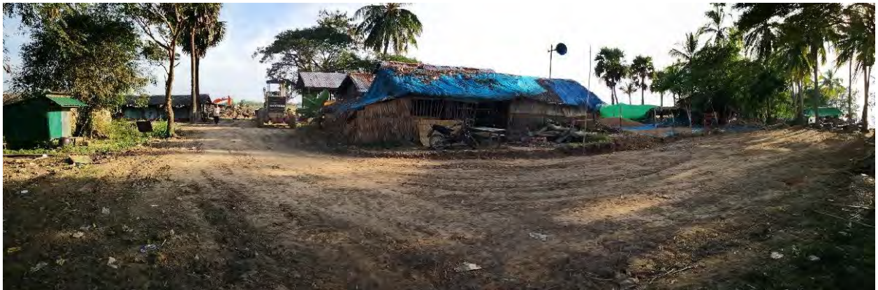
Existing access road from riverside to plant yard was widened and made good by MOC
